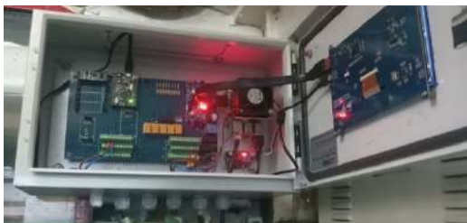
Figure 8. Main Monitoring Panel
